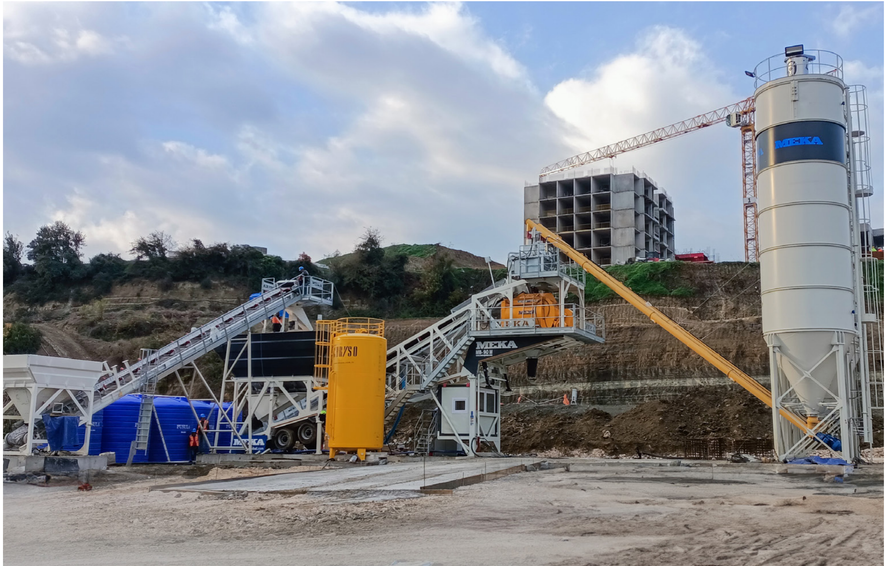
▲ MEKA Mobil Beton Santrali Hatay
